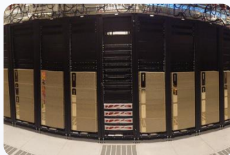
BERZELIUS SWEDEN DATA CENTER
